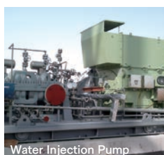
Water Injection Pump
