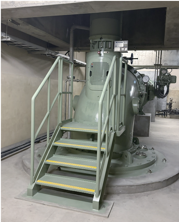
図3 1号雨水ポンプ外観 Fig. 3 Appearance of Pump
