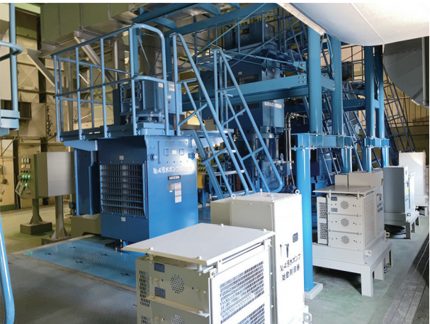
図5 No.4汚水ポンプ電動機外観 Fig.5 View of the No.4 motor
