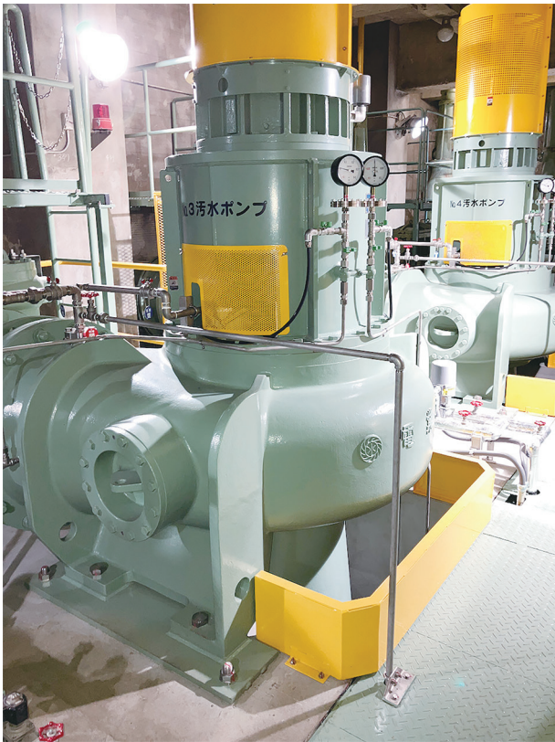
図4 No.3, 4汚水ポンプ外観 Fig.4 View of the pump
