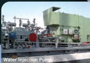
Water Injection Pump
