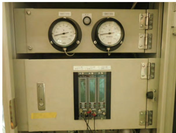
図6 機側盤 Fig.6 Monitoring panel
