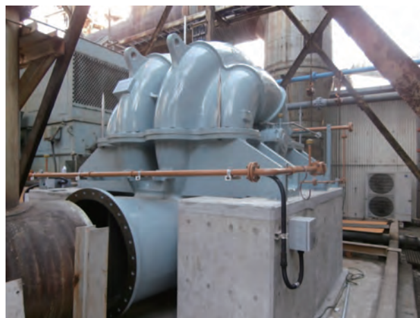
図8 ブロワ現地据付状態 Fig.8 View of blower at site
