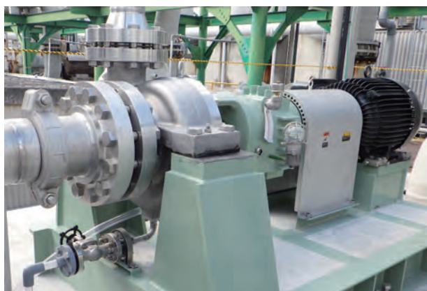
図8 増圧ポンプ外観 Fig.8 View of booster pump
